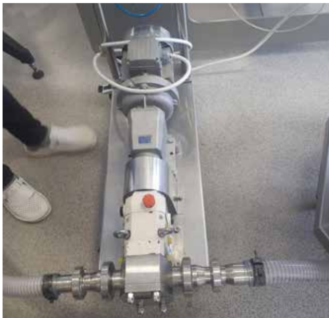
Pumped liquid - toothpaste, body scrubs, lotions creams Pump - LPX50-1 delivering 2 m 3 /h at 5 bar differential pressure
