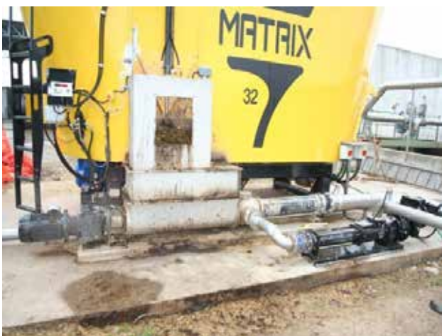
DHS-T and DN pump Transferring biomass to the digester with phase liquid injection.
